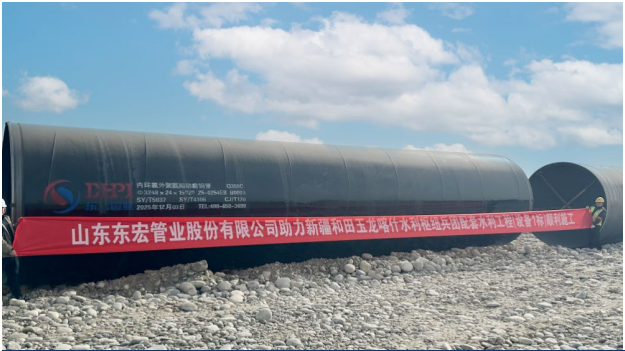
COROLLARY WATER PROJECT FOR XPCC OF HOTAN YULONG-KASHGAR WATER CONTROL COMPLEX, XINJIANG
